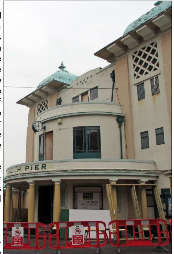
Photo taken on 11.10.12 outside the Penarth Pavilion , showing that work on the restoration is now well under way!
